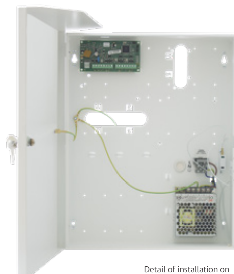
Detail of installation on metal cabinet
